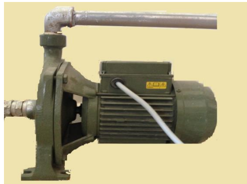
Figure 6.3 water pump no. 1
